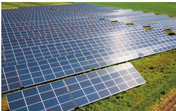
Ground-mounted solar panels.
